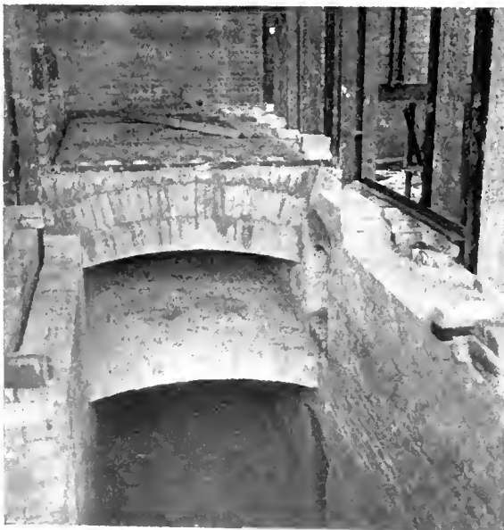
Draft is preheated in a regenerator shown here under construction. Part of the gases of combustion passes through upper passage and through vertical tubes and around which the air is circulated.
